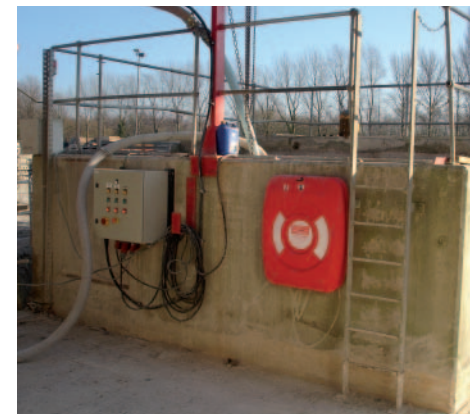
The waste water processing tank.
