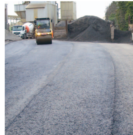
Low energy asphalt was trialled at Hanson's West Drayton asphalt plant in Middlesex before being used on the local road network
