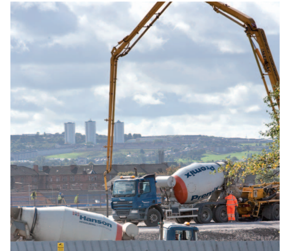
Shawfield concrete plant at Rutherglen is supplying concrete to the new Sir Chris Hoy Velodrome being built in Glasgow for the 2014 Commonwealth Games
